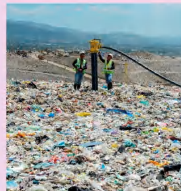
Methane is extracted at the Payatas landfill, Manila—the first in the Philippines to have the gas converted to energy, as part of a United Nations program.
